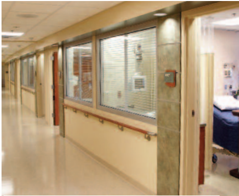
Vision Control® installed in borrowed lites at Lakeland Regional in Lakeland, FL
